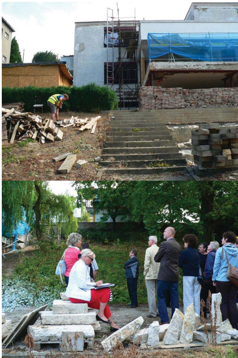
Fig. 41. Villa Tugendhat, Brno, architect Ludwig Mies van der Rohe (1929-1930), during restoration. Photo: Alex Dill.
