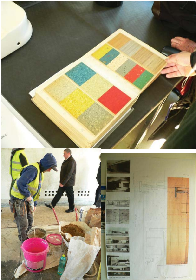
Fig. 43. Villa Tugendhat, Brno, architect Ludwig Mies van der Rohe (1929-1930), during restoration. Photo: Alex Dill.
