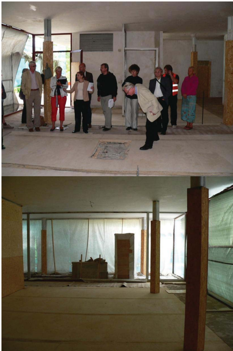
Fig. 42. Villa Tugendhat, Brno, architect Ludwig Mies van der Rohe (1929-1930), during restoration. Photo: Alex Dill.
