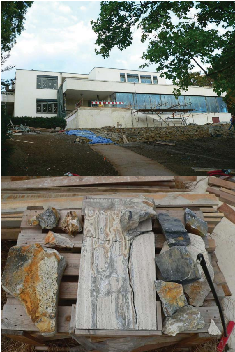
Fig. 40. Villa Tugendhat, Brno, architect Ludwig Mies van der Rohe (1929-1930), during restoration. Photo: Alex Dill.
