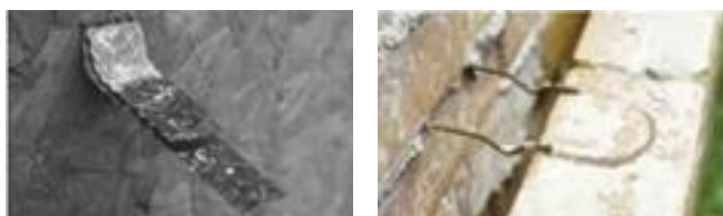
Fig. 6a: Ancore avariate prin coroziune Anchors damaged by corrosion
