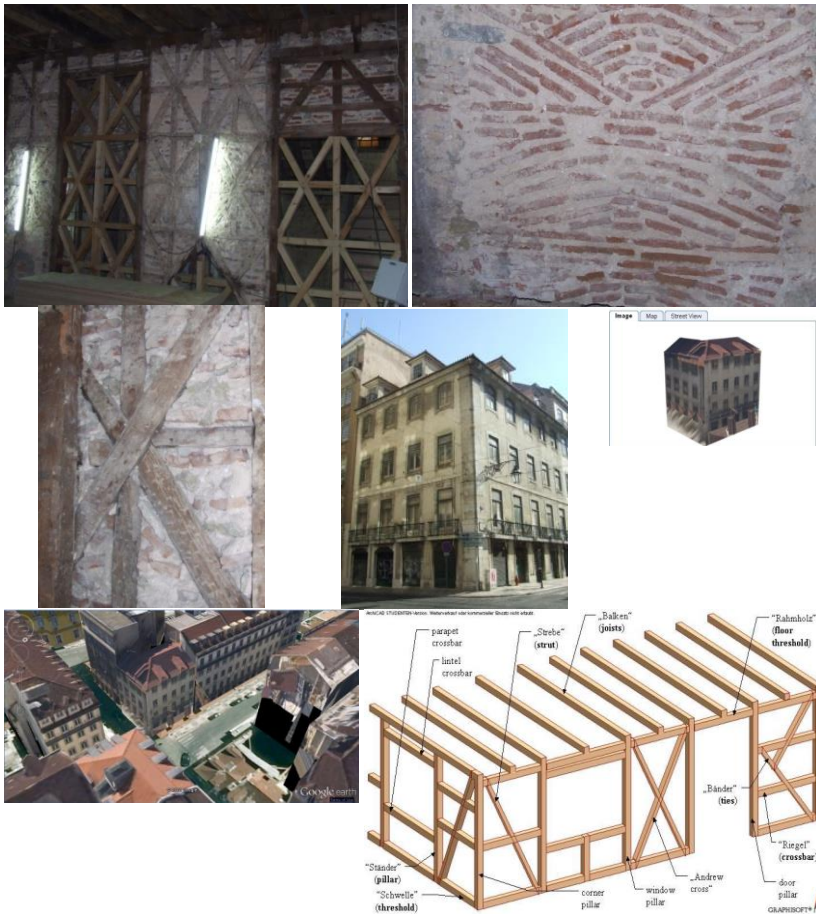
Fig. 24. Google Earth in Lisbon. A typical “pombalino” half timbered building (interior view of the “pombalino wall” versus the ancient wall, interior detail and sketch) modeled in Google Earth with BuildingMaker. For such buildings a different level of detail is necessary to see the structure. Photos: M. Bostenaru, 2008, models in BuildingMaker, M. Bostenaru, 2012. Sketch from Bostenaru (2004).
