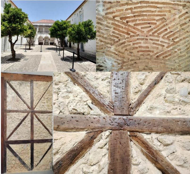
Fig. 46. A typical “pombalino” half timbered building intervention on Casa da Cerca in Almada, on the other side of the Tejo as Lisbon: view of the house, view of the ancient 15 th century wall and view of the “pombalino” wall. Note the same typology for both walls as in Fig. 23. Photos: M. Bostenaru, 2023.
