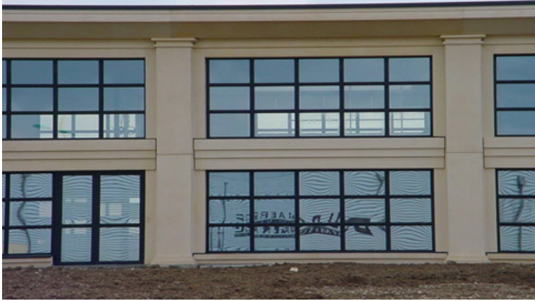
Fig. 1. In the reflections on the ground floor one can notice a lack of flatness from the objects reflected acting as guiding lines. At the first floor, due to lack of guidance lines (only sky is reflected), glass seems much more flat. Note: both ground floor and first floor have exactly the same glass structure but apparently they look very different.
