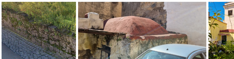
Fig. 14. Buildings – Functional errors. Source: Authors' archive.
